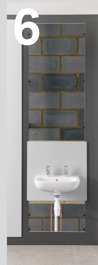
06 Once all the units are in position, connect the plumbing and services.
