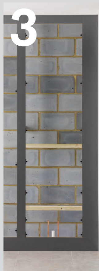
03 Attach fixing clips to the inside edge of the vertical flashgaps, repeat process on back face of panels.
